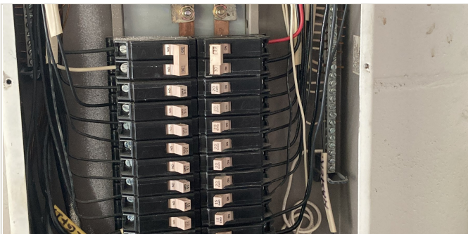
Electrical box with panel off
